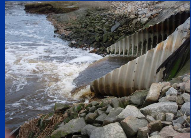
Hanging Culvert, Cascade Brook, ME
