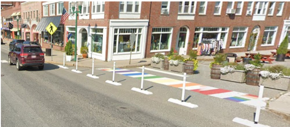
Ellsworth Route 1/3 - Using Tuff Curb to Block Town Way and Protect Crosswalk
